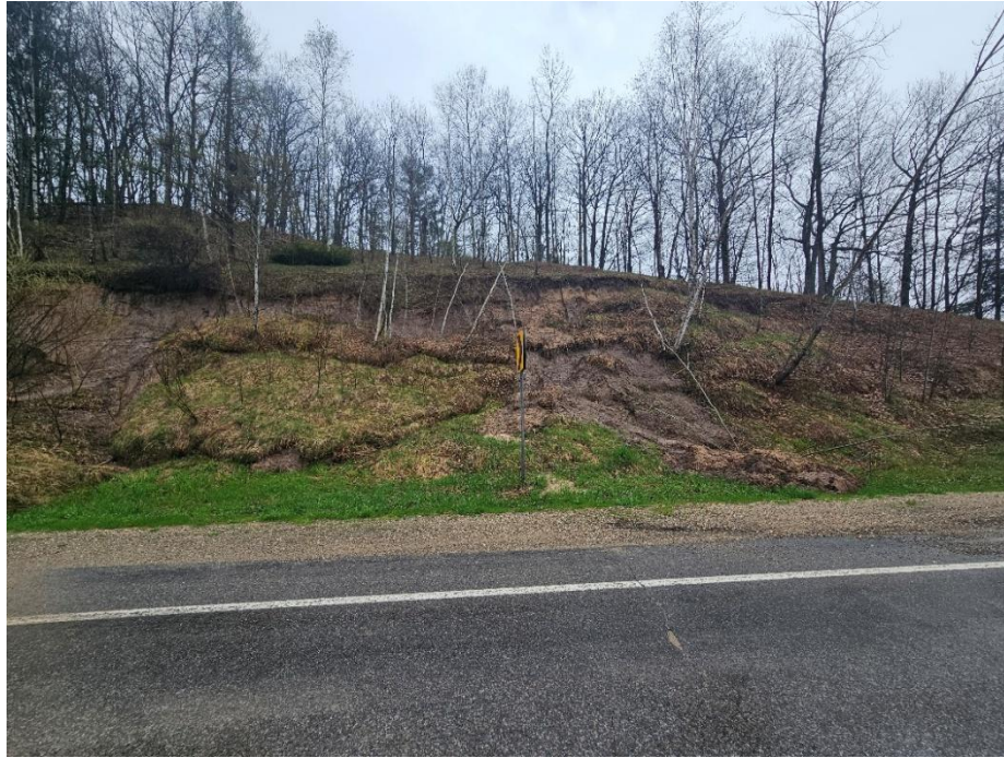
Photograph #1: Slope failure of cut slope adjacent to the north bound lane. View is to the east. (April 2026)
