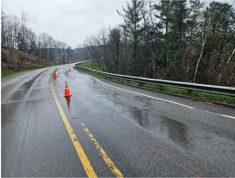
Photograph #3: Cracking in southbound lane near the north end of the area of concern. (April 2026)
